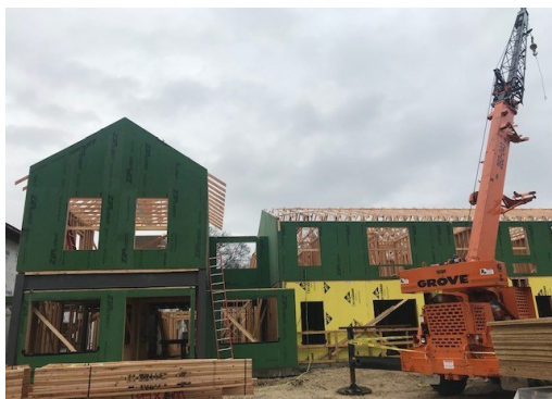
Our new entrance and second floor are starting to look like a real building
