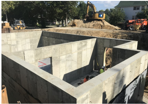
The foundation for the basement, including our new storm shelter is completed
